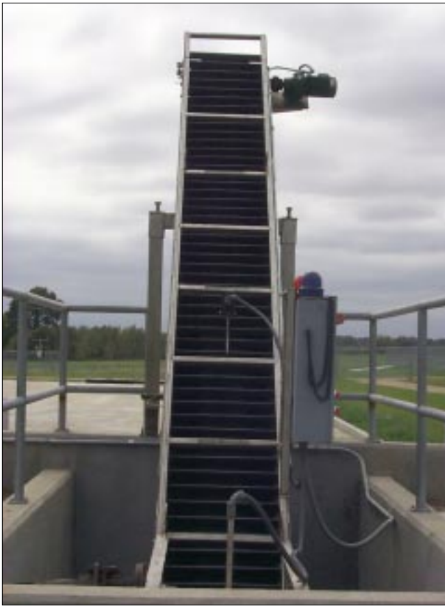
An in-channel flighted conveyor separator.
