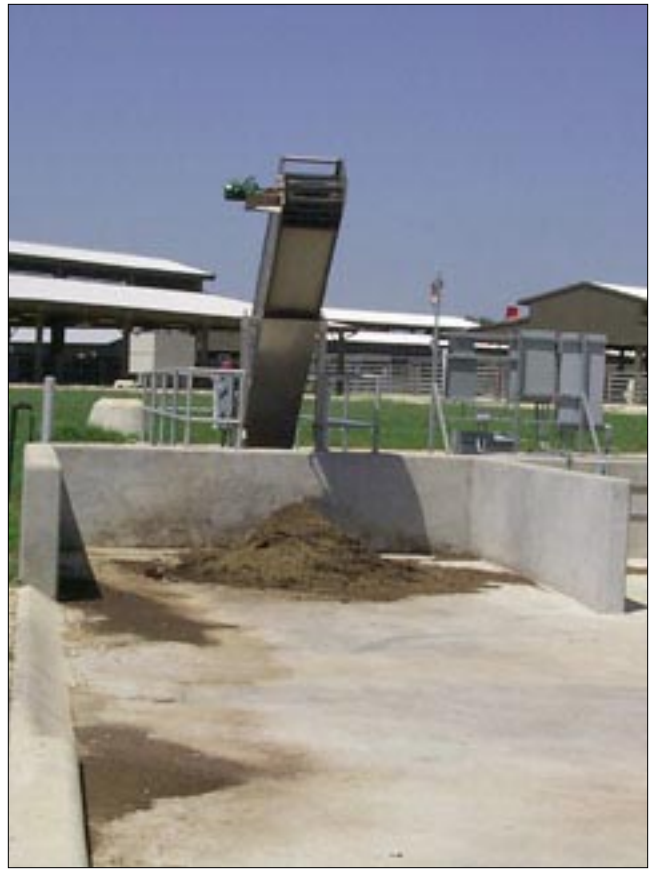
The discharge end of an in-channel flighted conveyor separator.
